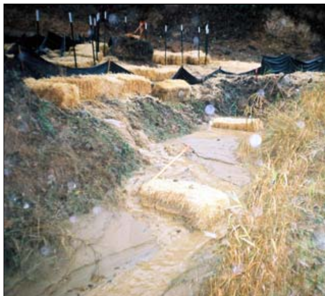
Heavy rain can blow out conventional stormwater treatment measures.
