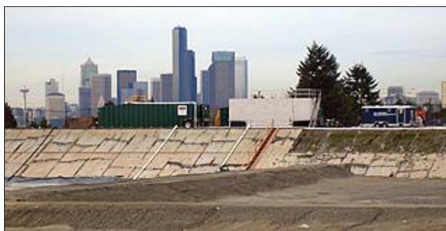
A chitosan-enhanced sand filtration system is being used to treat runoff from construction work at the Beacon Hill Reservoir.
