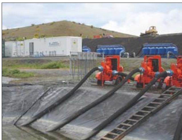
The Port of Seattle is using a chitosan-enhanced sand filtration system on its Third Runway project. More than 100 million gallons of stormwater have been treated since November 2005. Images courtesy of Clear Water Compliance Services
